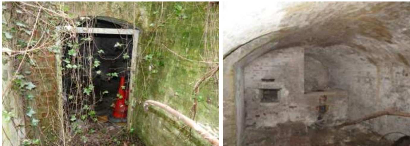
Fig 8 The old bakehouse. Left: Entrance doorway 2023; Right: Interior (c 2010). This room is not accessible from the inside of Upton House.
