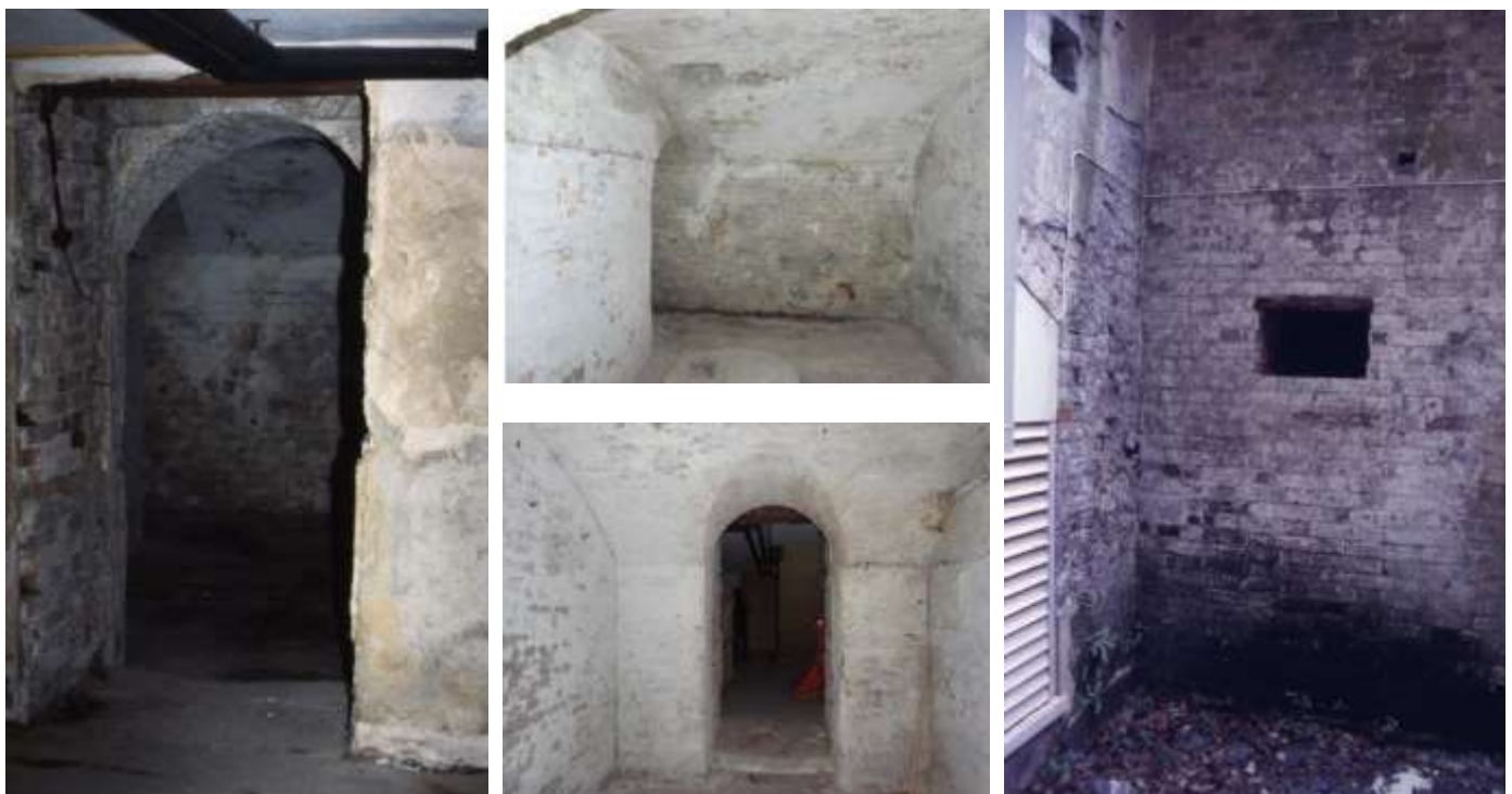
Fig 7 The ‘bat cave’ (Left to Right): Entrance from lobby to squash court (prior to fitting of wooden gate); Top: Interior: Lower: Entrance from inside; Right: bat access hole in nearby wall (adjacent to room holding central heating boilers).
